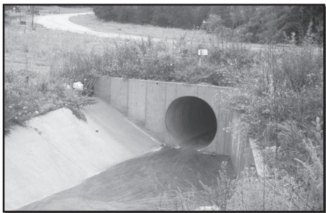
Most storm drains deliver stormwater directly to surface waterbodies without treatment.
